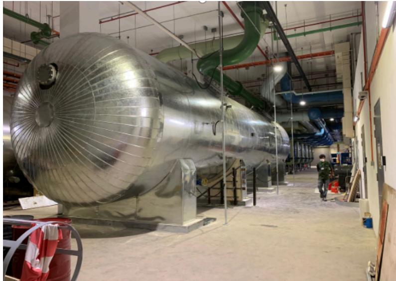
Insulated tank - installed condition
